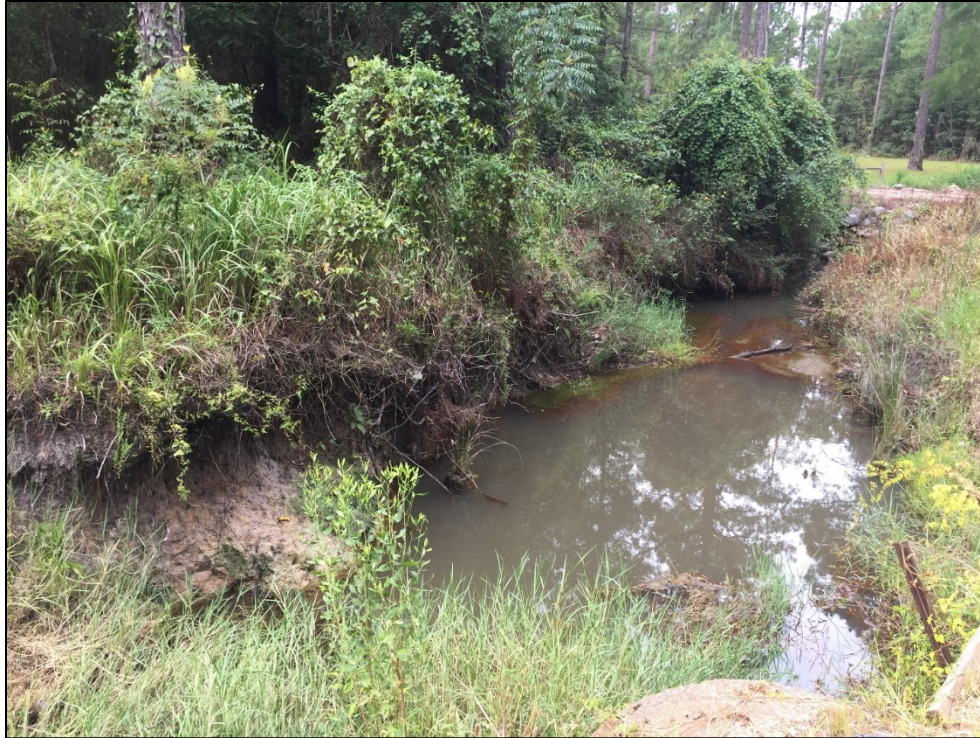
Figure 4.12 Bank scour associated with a road culvert crossing
