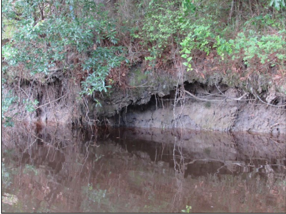
Figure 3.26 Photo of typical bank failure and undercutting in the upper reaches of the Watershed (Photo Credit Bret Webb)
