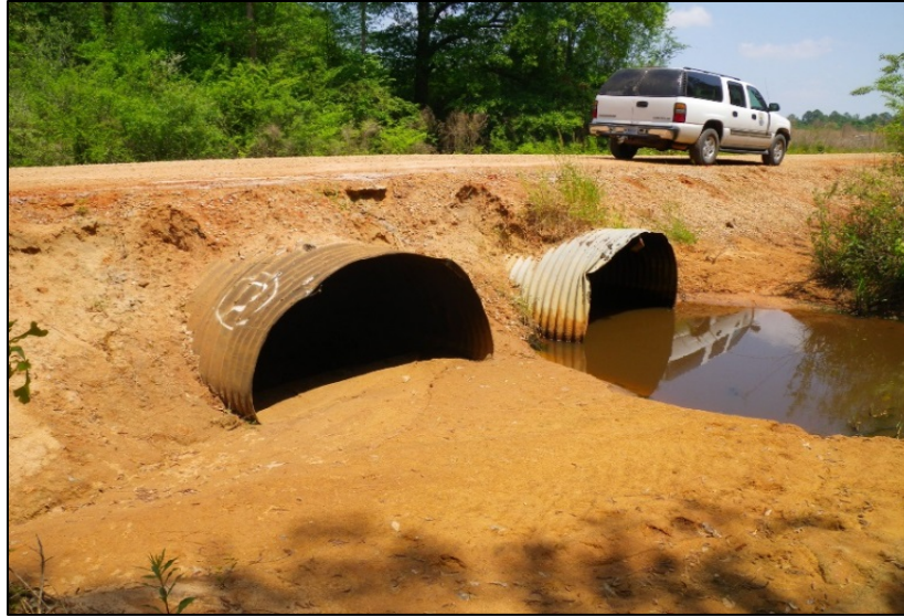
Figure 6.15 Unpaved road-stream crossing sedimentation
