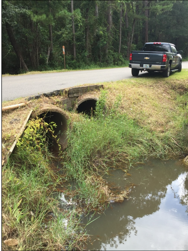
Figure 4.13 Elevated and clogged culvert crossing preventing upstream migration of aquatic organisms
