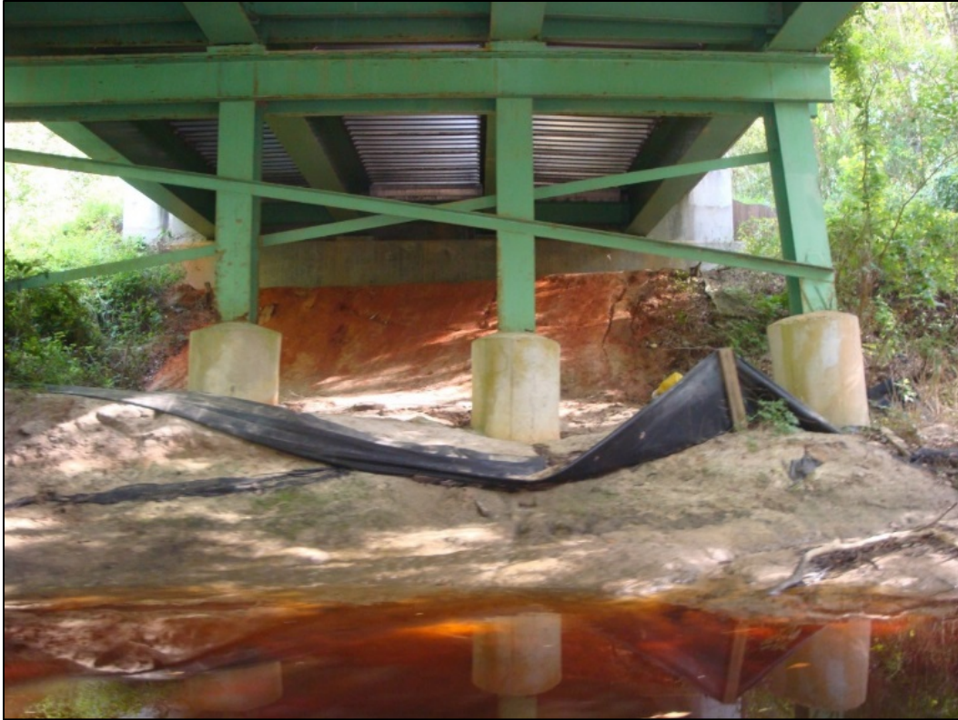
Figure 4.9 Inoperative BMP along upper Bayou
