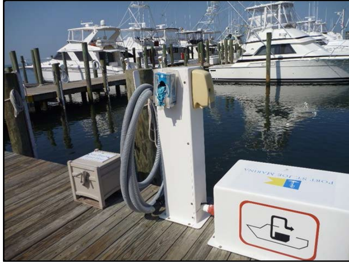
Figure 6.24 Boat pump out station. Source: FDEP Clean Marina Program
