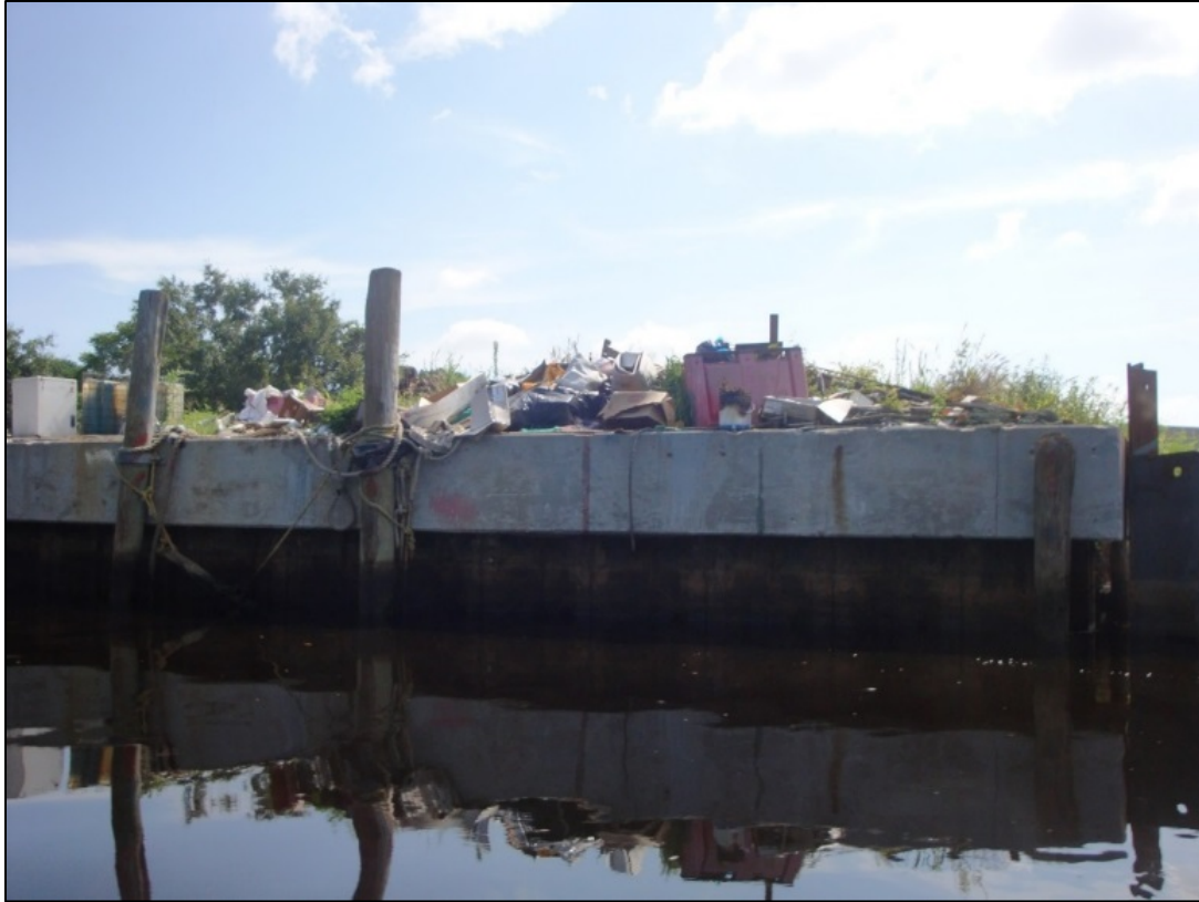
Figure 4.3 Trash stacked along Bayou La Batre with no containment
