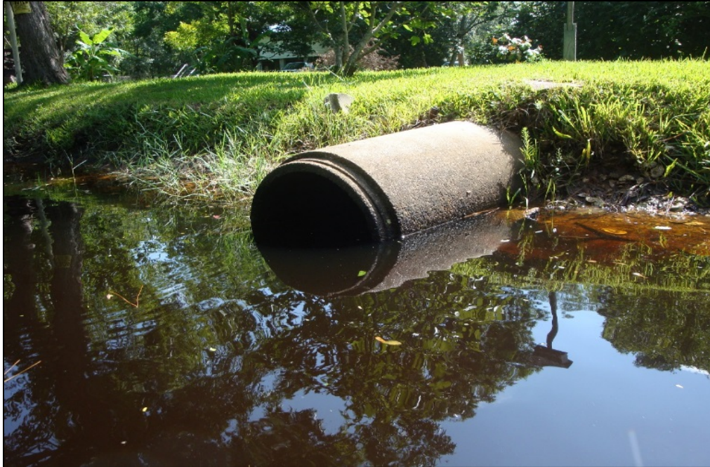
Figure 6.1 Existing untreated stormwater discharge in Bayou La Batre
