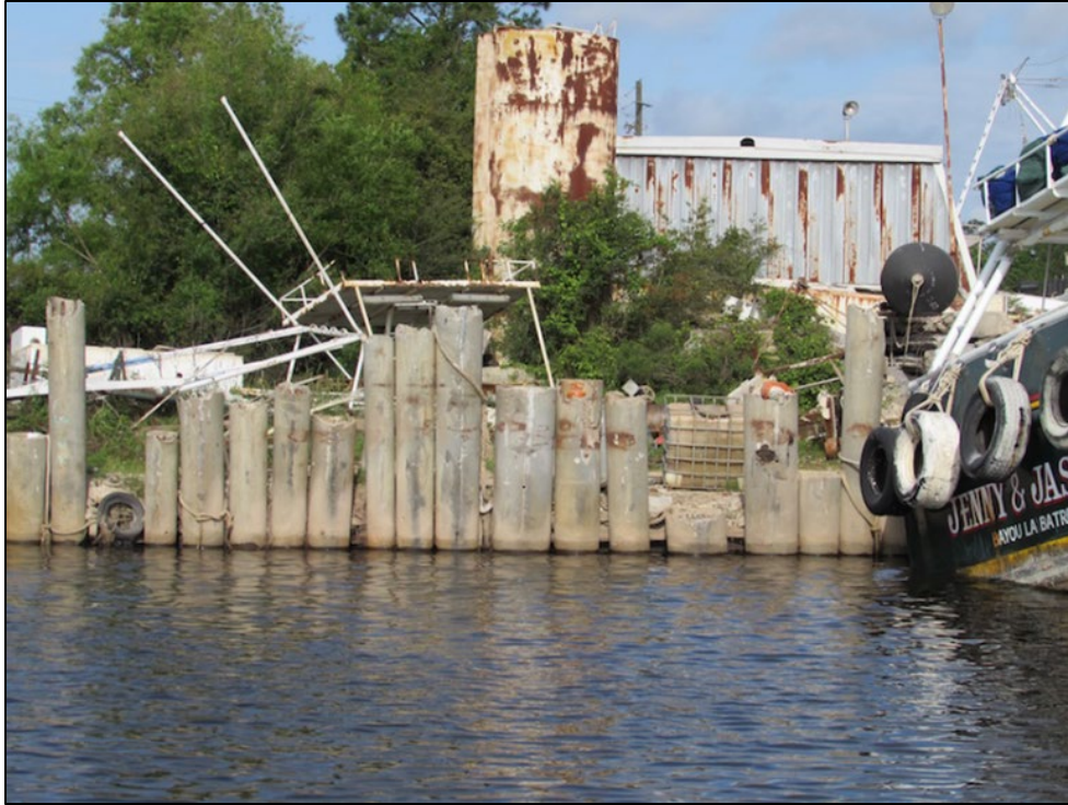
Figure 3.28 Typical example of failing or failed armored shoreline with upland erosion (Photo Credit Bret Webb)
