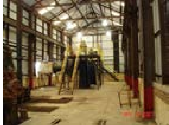
Figure 7.14: Storm Water Pump House
