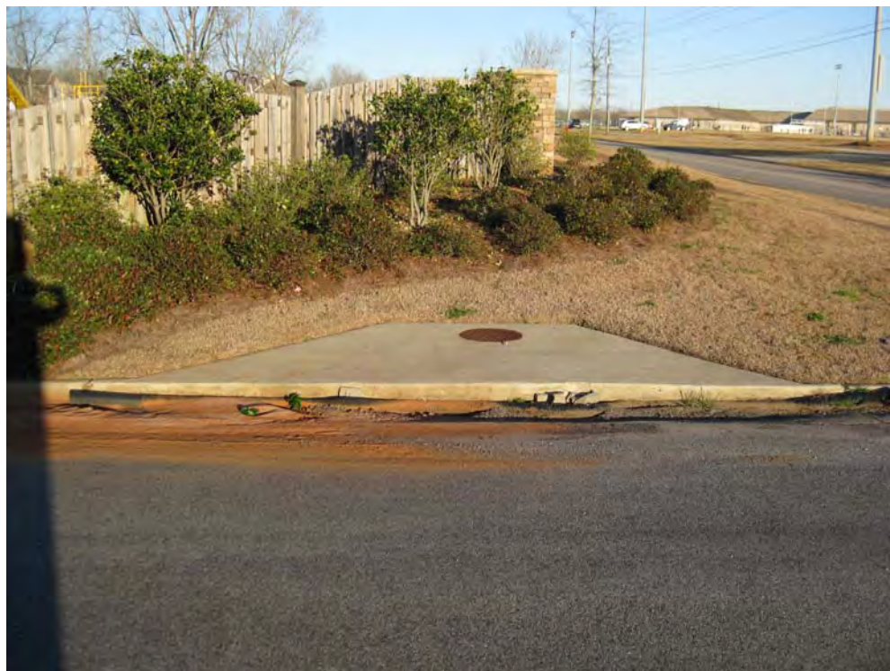
Figure 4-19. Sediments from Construction Sites Entering Drain Outlet
