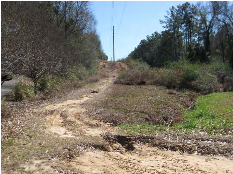
Figure 4-21. Erosion Occurring within a Power Line Right-of-Way
