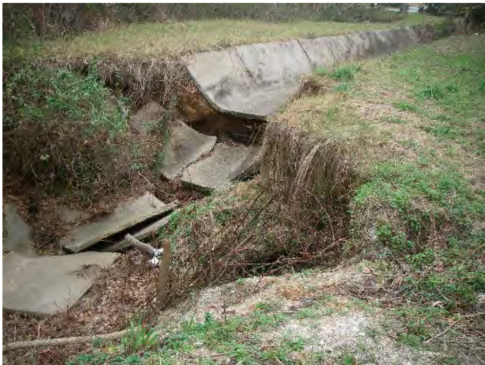
Figure 6-54. Example of Erosion Caused Damage
