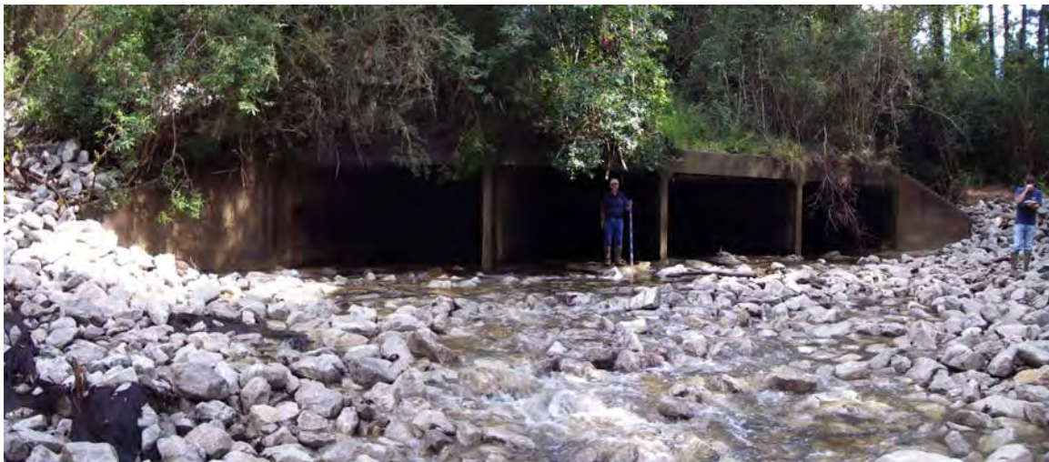
Figure 4-6. Riprap Downstream of I-10 Bridge Crossing on D'Olive Creek to Protect Against Head-Cutting Induced Erosion
