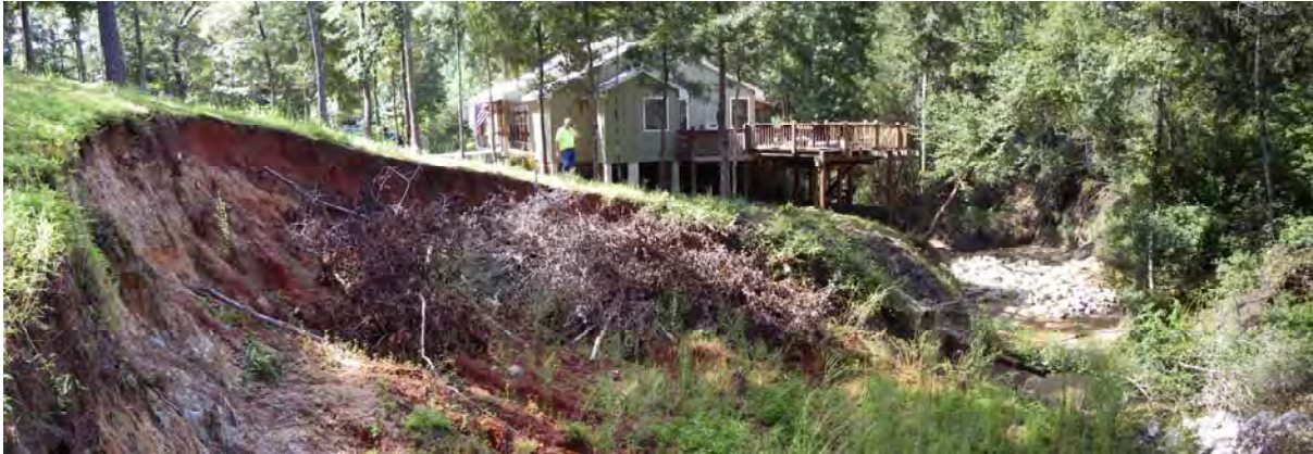
Figure 3-5. Example of Home Threatened by Mass-Wasting of Streambank from March 2009 Storm Event
