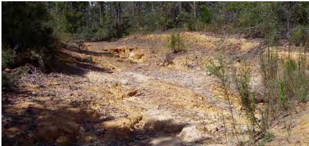
Figure 5-22. Eroding unpaved road north of tributary TCB. Site U46.
