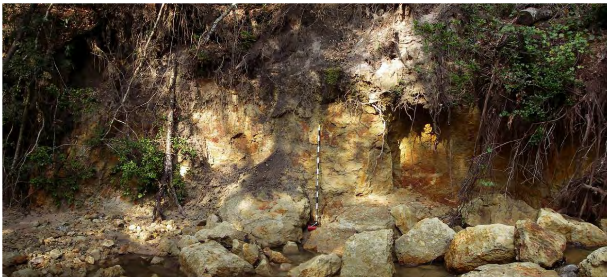
Figure 5-7. Erosion by block failure observed at DA22 and DA34. Site DA22
