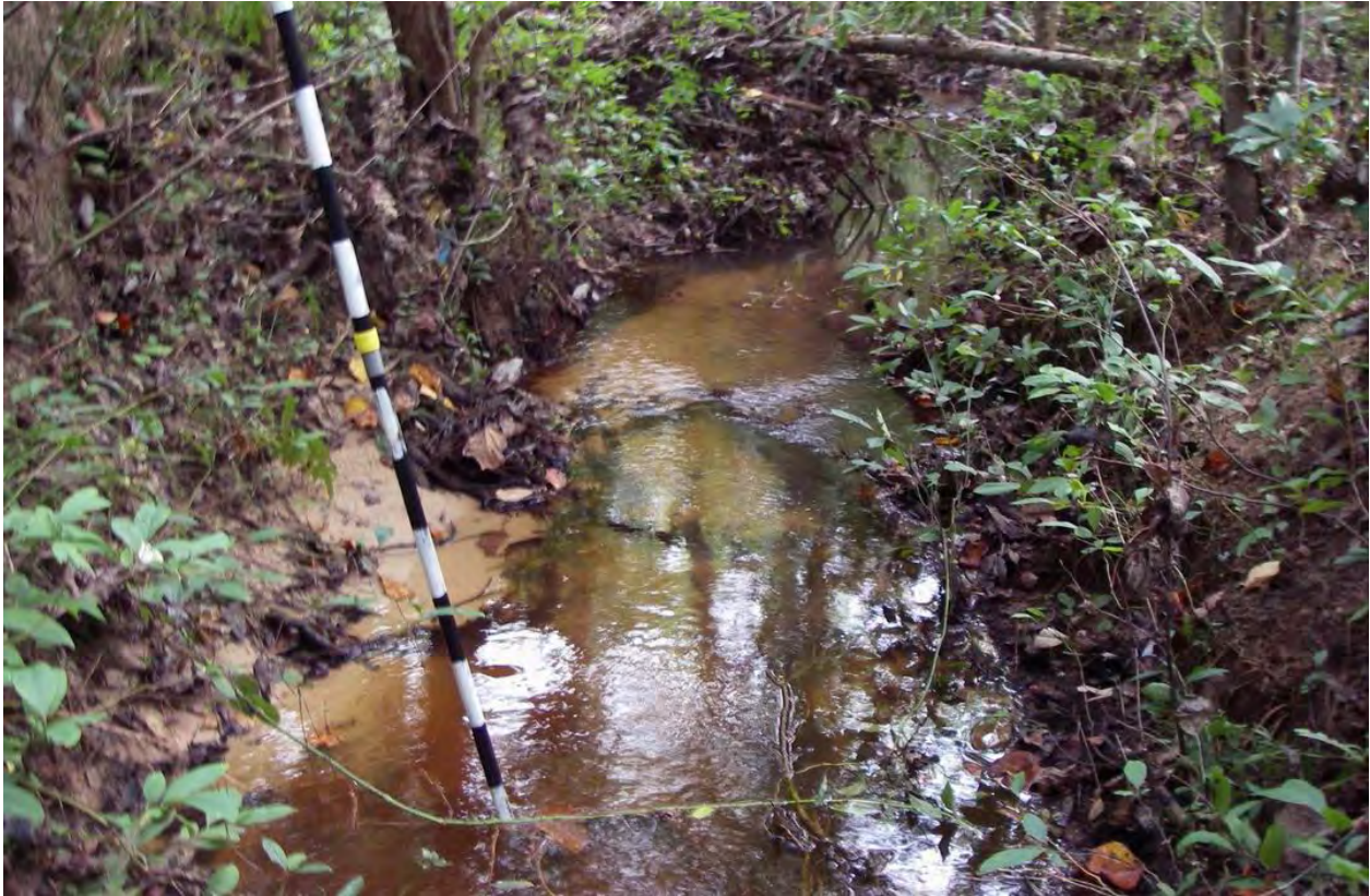
Figure 5-11. Stable reach DC. Site DC7.
