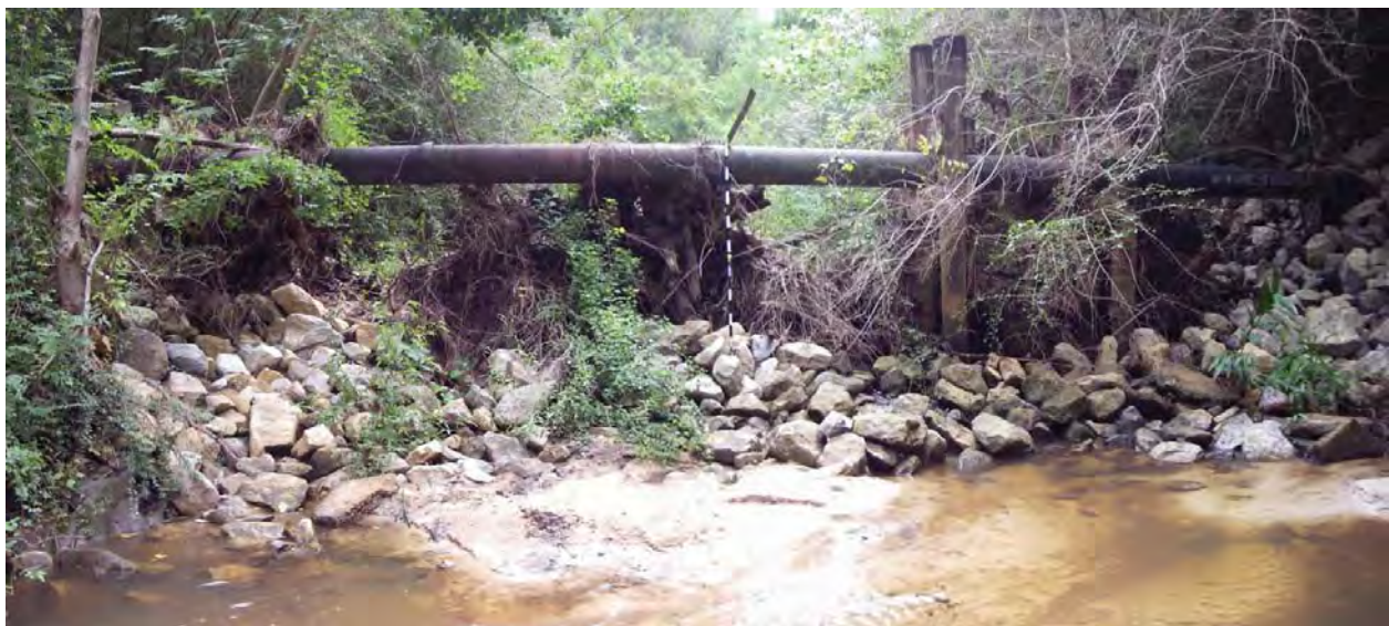
Figure 4-6. Woody debris jam formed on sewage pipeline crossing. Site T18.
