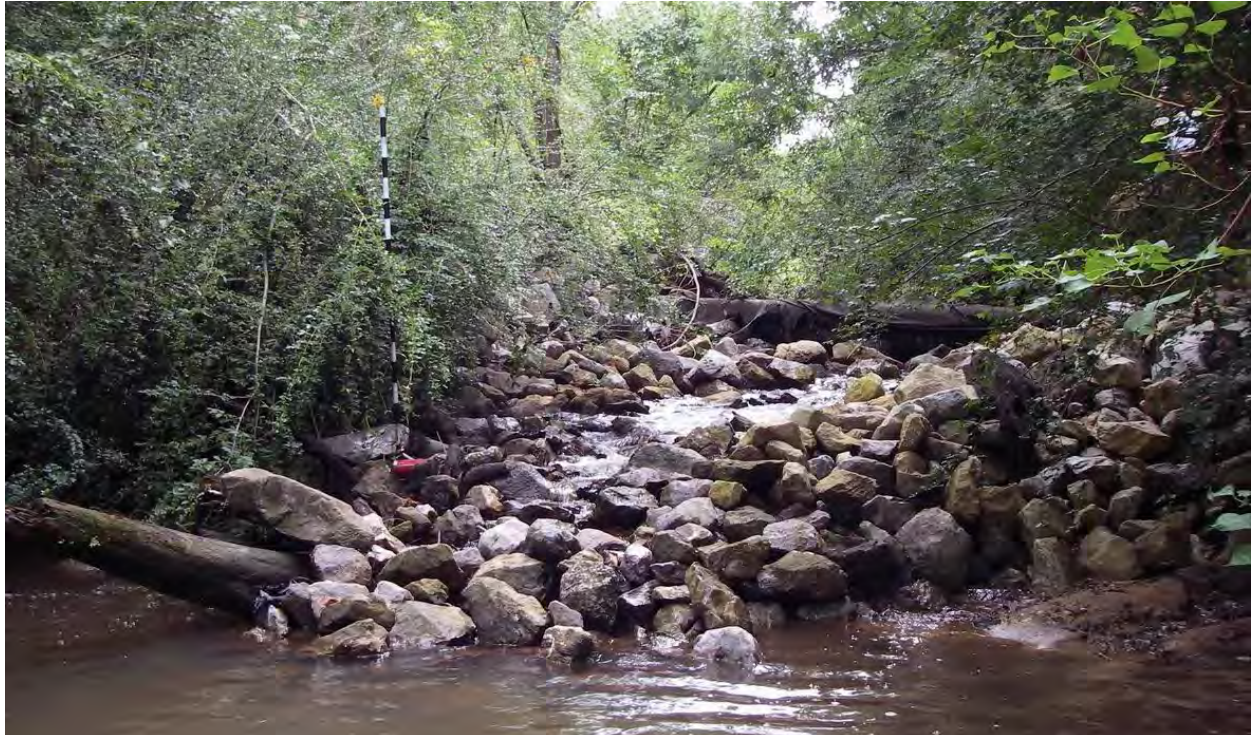
Figure 5-16. Typical riprap grade control protecting sewage pipeline on Tiawasee Creek. Site T23.
