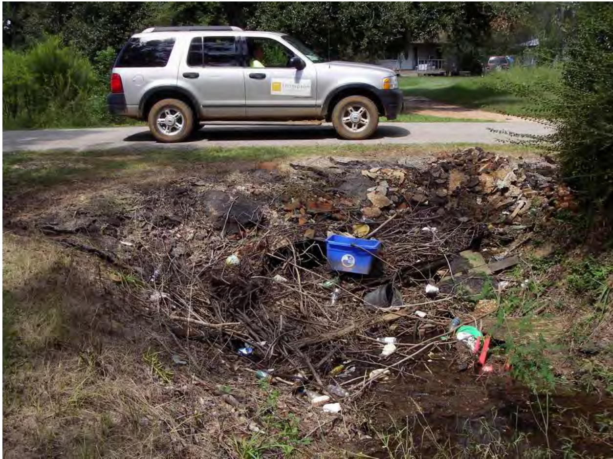
Figure 4-7. Culvert blocked by debris. Site TCC1.
