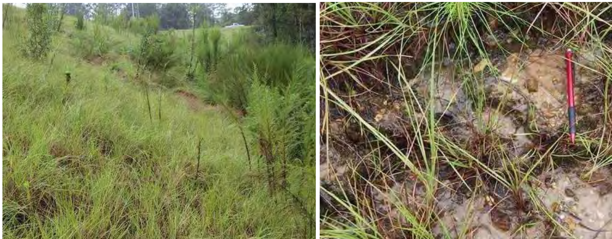
Figure 4-16. Not fully established grass protection. Note pooling runoff. Site U1.
