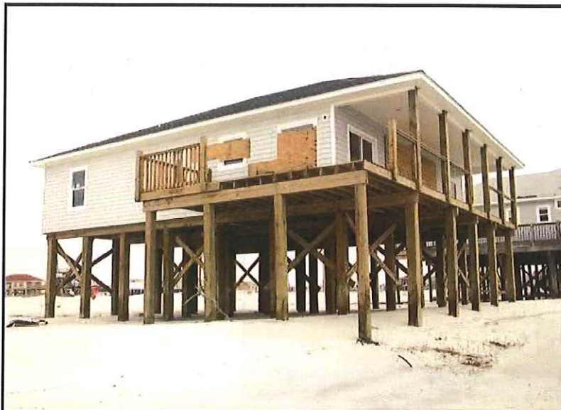
Figure 6-10. DAUPHIN ISLAND, ALABAMA: Successful pile foundation following Hurricane Katrina. The foundation supported the elevated home even after scour and erosion removed several feet of soils. (Source: FEMA 549)
