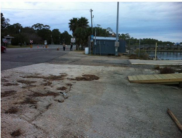
Photo: Flood prone area near ferry. Credit: T. Webler 2012
