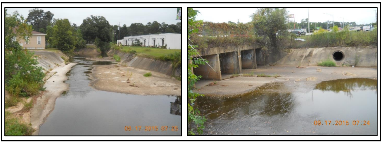
Figure 5.2.36: General views of Moore Creek upstream from U.S. Highway 90 (left) and downstream from U.S Highway 90 (right)
