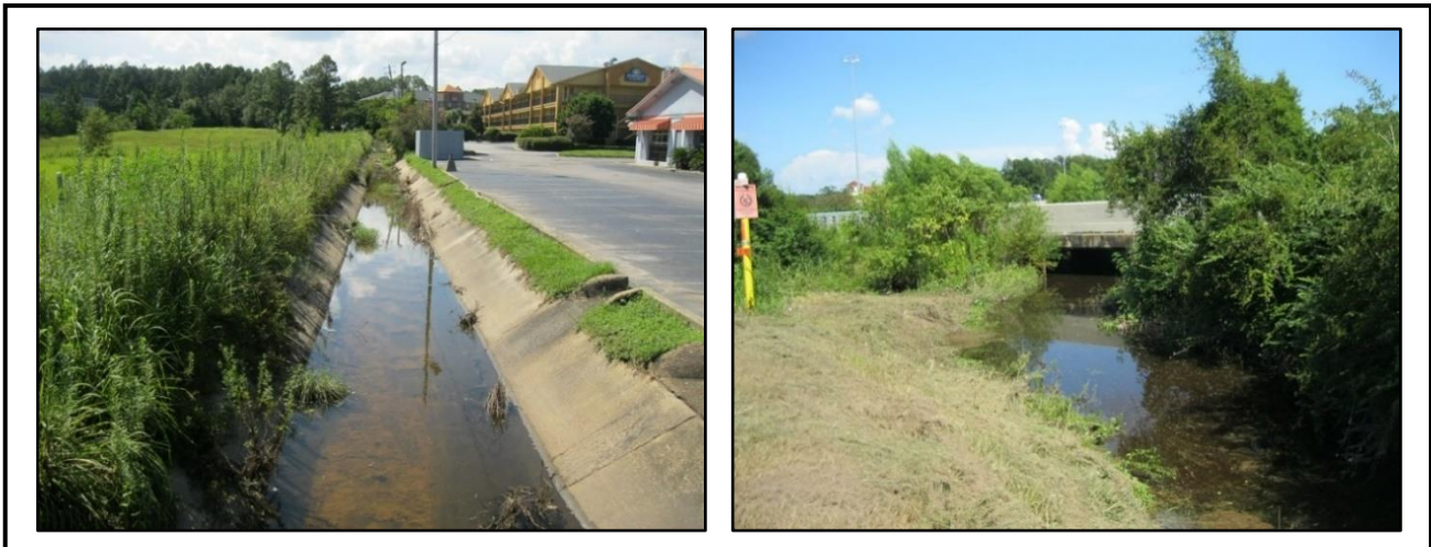
Figure 5.2.104: Concrete drain (left) and mowed bank (right) show ponded water in the unnamed tributary of Rattlesnake Bayou (Upper Rattlesnake Bayou - Service Road)
