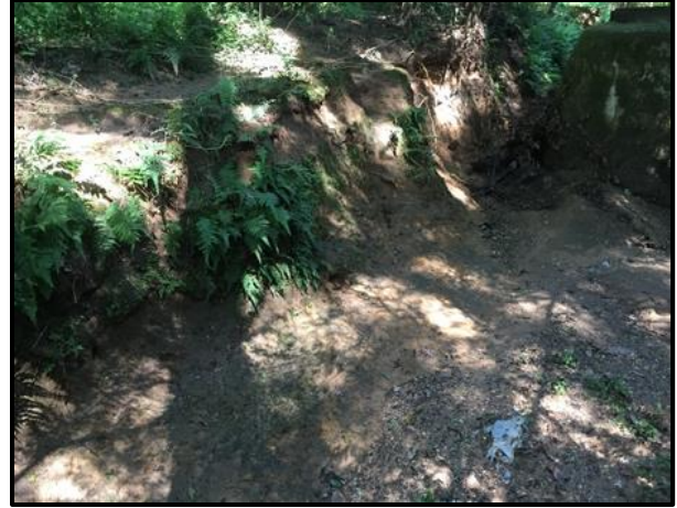
Figure 5.2.54: Example of eroding banks (Spring Creek – Cottage Hill Road to Woodland Road)
