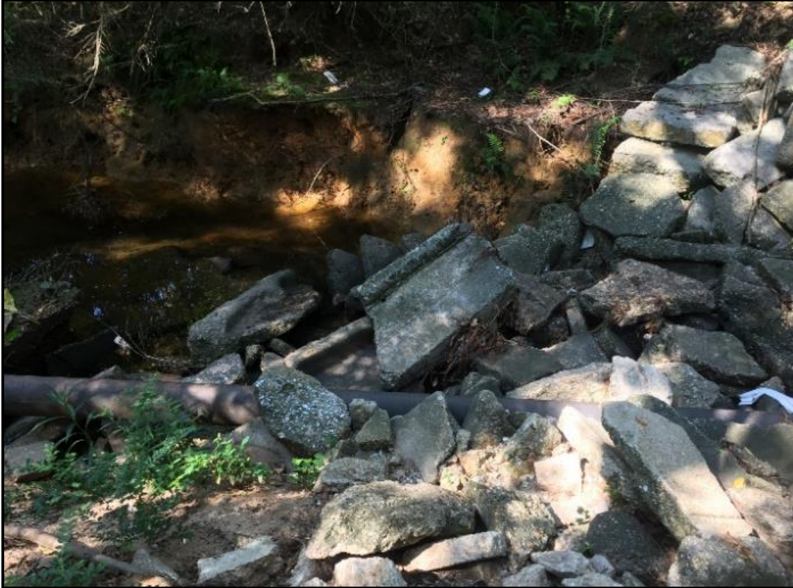
Figure 5.2.50: Concrete riprap and eroding bank interface with visible sewer line (Spring Creek – Cottage Hill Road to Woodland Road)
