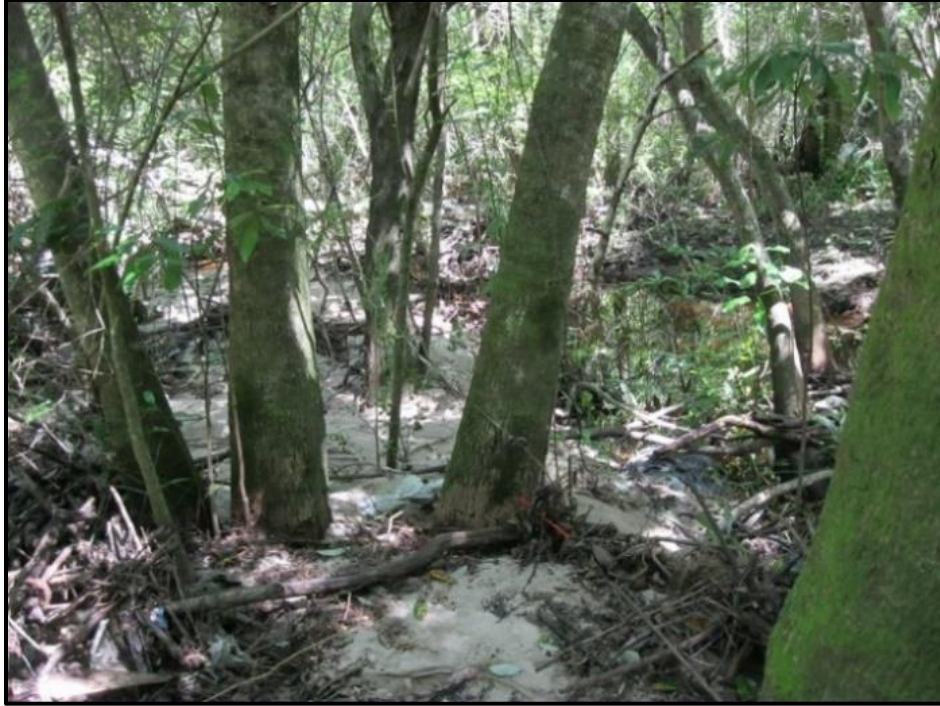
Figure 5.2.112: General view of system aggradation and reduced channel capacity (Rattlesnake Bayou - Business Parkway)
