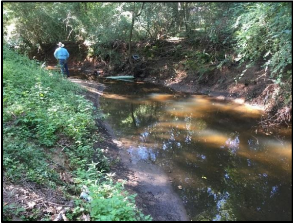
Figure 5.2.51: Example of eroding banks (Spring Creek – Cottage Hill Road to Woodland Road)
