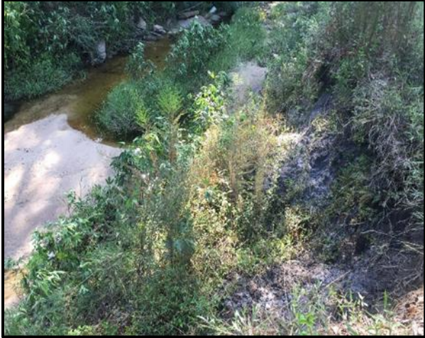
Figure 5.2.57: Sloughing banks and resulting sedimentation in channel (Spring Creek – Timberland Drive to Longleaf Drive)
