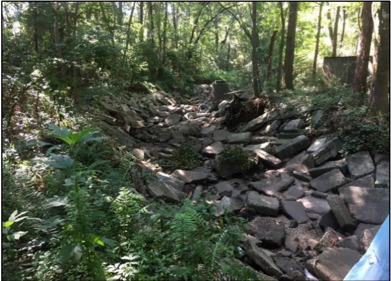
Figure 5.2.49: Concrete lined channel with exposed manhole (Spring Creek – Cottage Hill Road to Woodland Road)
