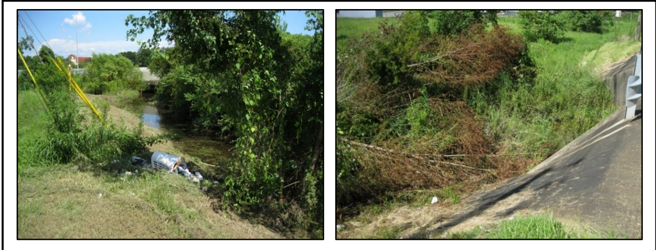
Figure 5.2.103: General view of grass clippings, garbage, and tree debris discarded in the unnamed tributary of Rattlesnake Bayou (Upper Rattlesnake Bayou - Service Road)
