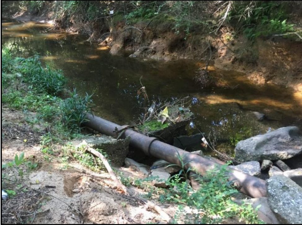
Figure 5.2.46: Example of an exposed sanitary sewer line in Spring Creek
