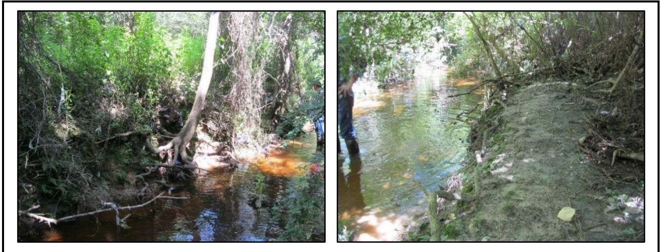
Figure 5.2.106: General view of a somewhat stable bank (left) and a stable bank with deposition bench (right) downstream from Motel Court (Upper Rattlesnake Bayou - Motel Court)
