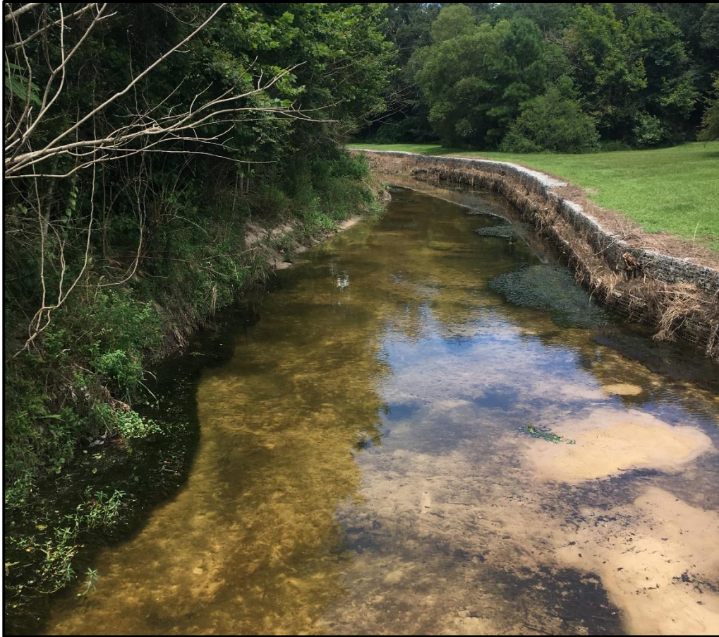
Figure 5.2.76: Example of sediment deposition and gabion armoring (Spring Creek – at Halls Mill Road)
