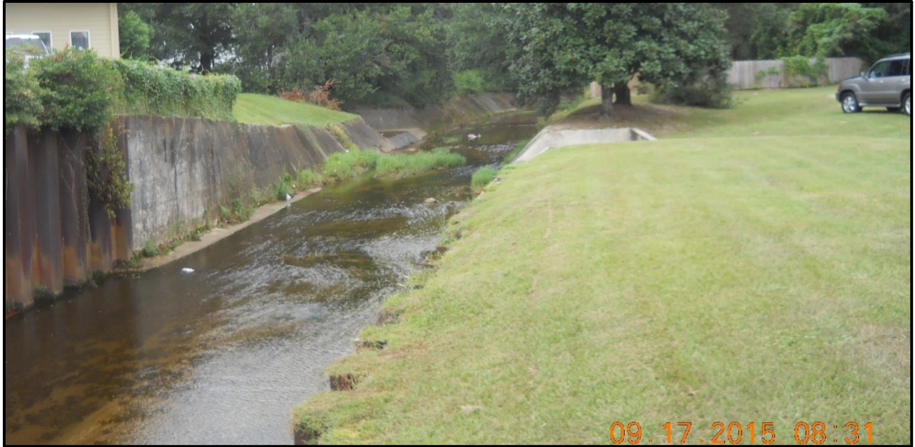
Figure 5.2.93: General view of West Bolton Branch upstream of Azalea Road
