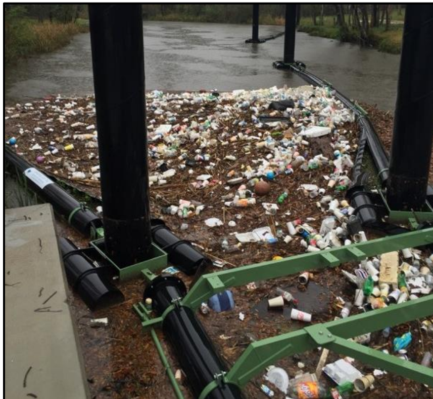
Figure 7.2.1: General view of the East Eslava Creek litter trap
