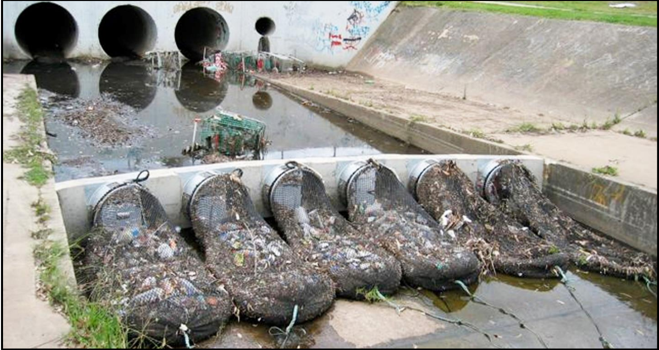
Figure 7.2.3: Example of stormwater pipe screens (Photo Credit: Storm Water Systems, 2015)
