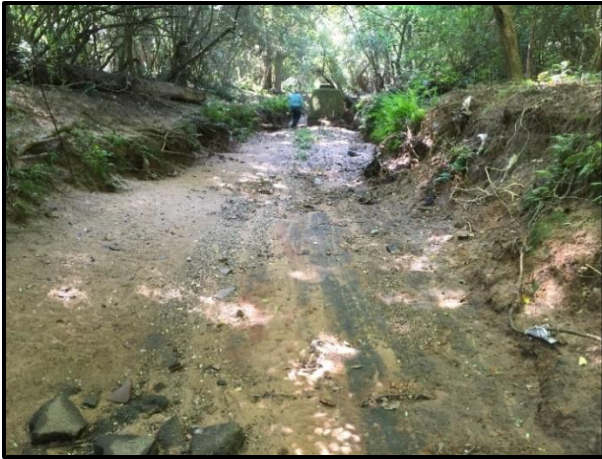
5.2.52: Eroding banks, instream deposition, and susceptible manhole (Spring Creek – Cottage Hill Road to Woodland Road)
