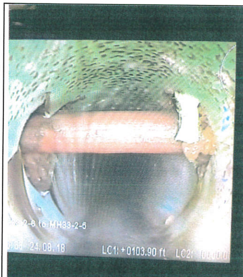
Pictured: Video shot by Water and Sewer Department of a sewer line showing conduit puncturing sewer line.
