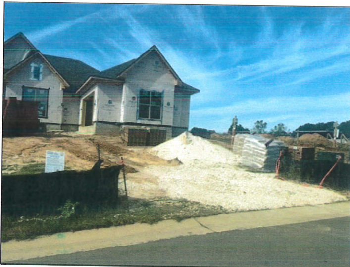
Pictured: Example of Fairhope's minimum BMP requirements on development projects: silt fence and construction entrance
