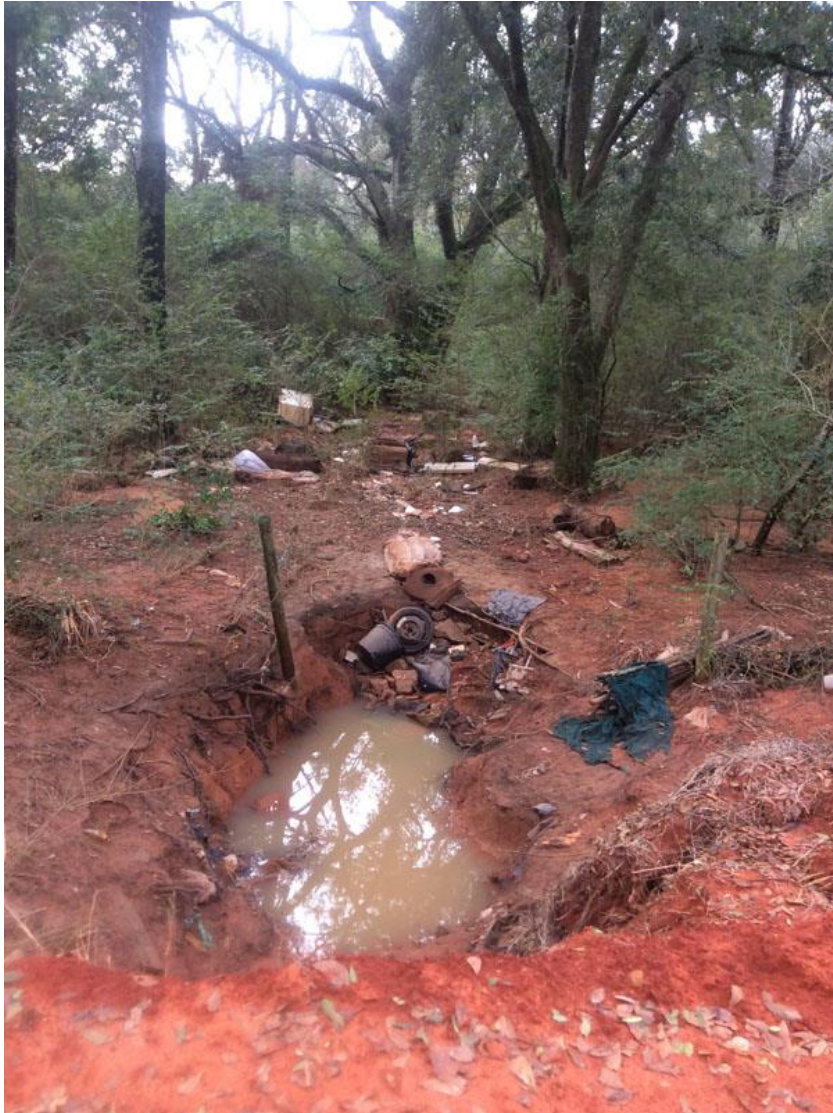
Figure 3.43 Heavily degraded drainageway in upper Eslava Branch. (Note: The green shrubs are mostly invasive Chinese privet)
