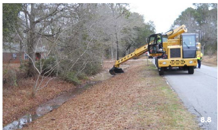
Figure 8.4: Trash in Muddy Creek; Figure 8.5: Example of public awareness signage; Figure 8.6: Fowl River community cleanup event held in 2015; Figure 8.7: Recently cleared ditch; Figure 8.8: County maintenance crew at work
