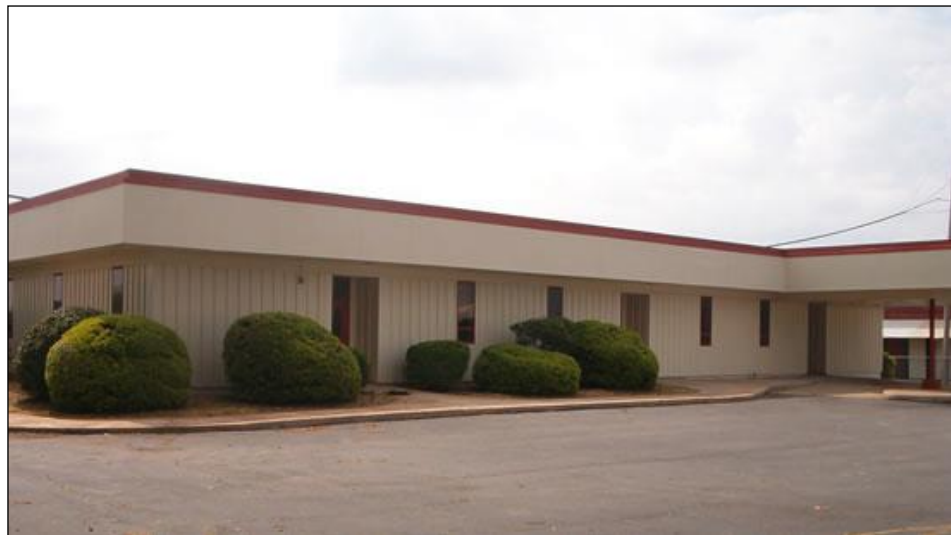
Inappropriate flat roof
