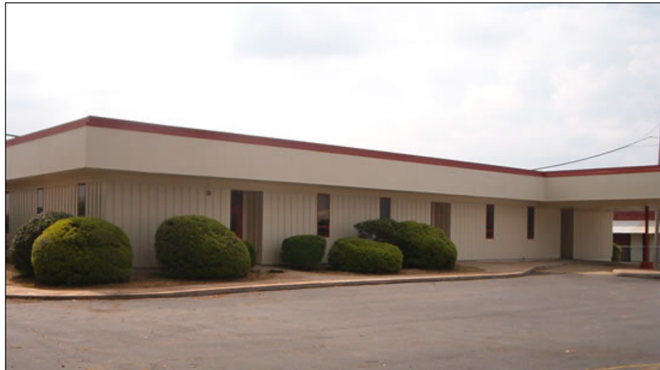
Inappropriate flat roof
