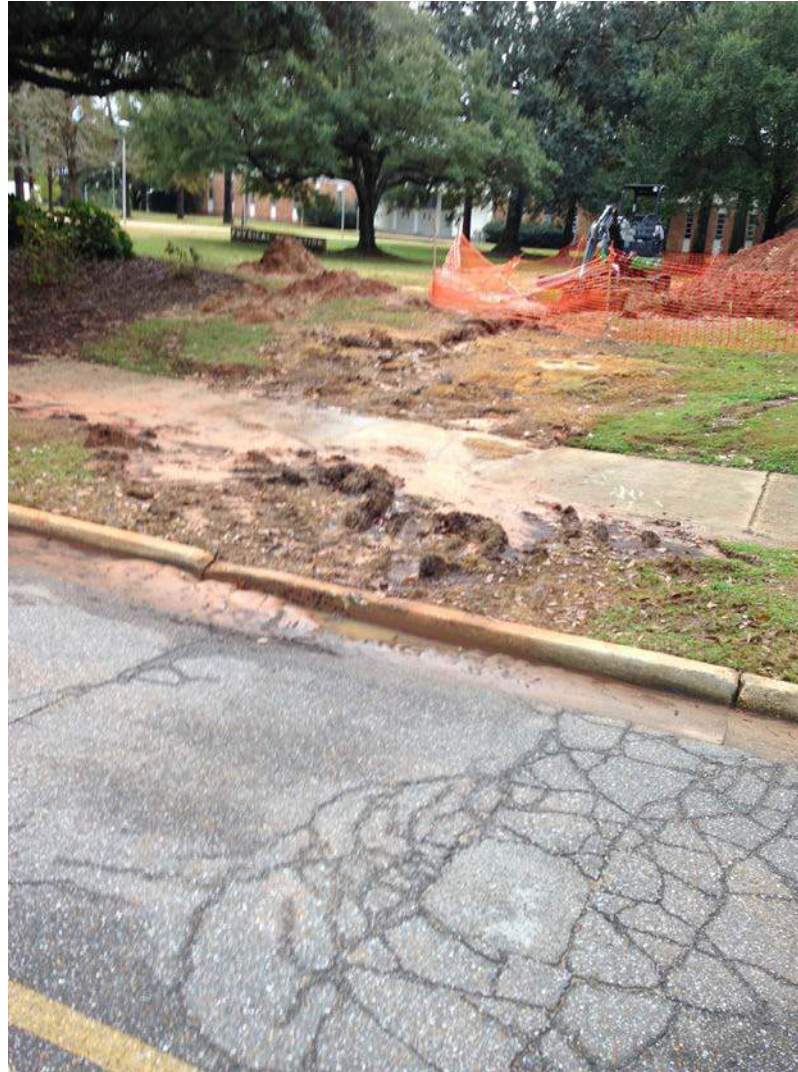
Figure 3-27 Eroded sediments from active utility construction site without erosion control entering roadway stormwater system connecting to Three Mile Creek, orange fence is for construction site safety, not erosion control (Location: USA Campus)
