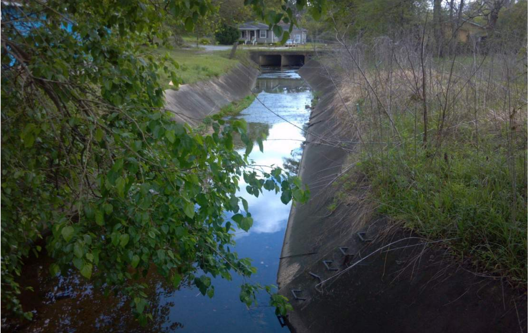
Figure 3-10 Concrete lined channel on Toulmins Spring Branch prohibits infiltration increasing stormwater runoff volumes and pollutant loads to Three Mile Creek, degrading water quality and habitat (Location: Toulmins Spring Branch downstream of Prichard Avenue)
