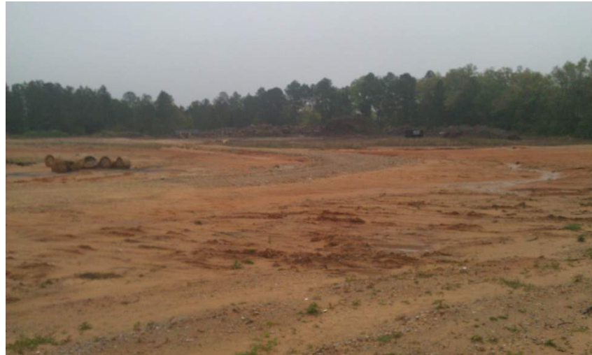
Figure 3-24 Undeveloped, exposed site near Cody Road and Zeigler Road with no construction site BMPs releases sediment and turbidity to Three Mile Creek, degrading surface water quality and habitat
