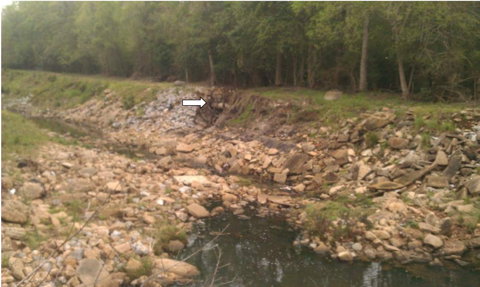
Figure 3-15 Exposed sanitary sewer pipe in Twelve Mile Creek from side stream erosion increasing the risk of a sanitary sewer leak into Three Mile Creek.
