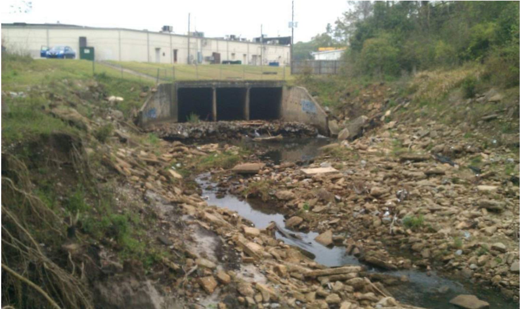
Figure 3-14 Erosion downstream of University Blvd in Twelve Mile Creek which flows into Three Mile Creek.
