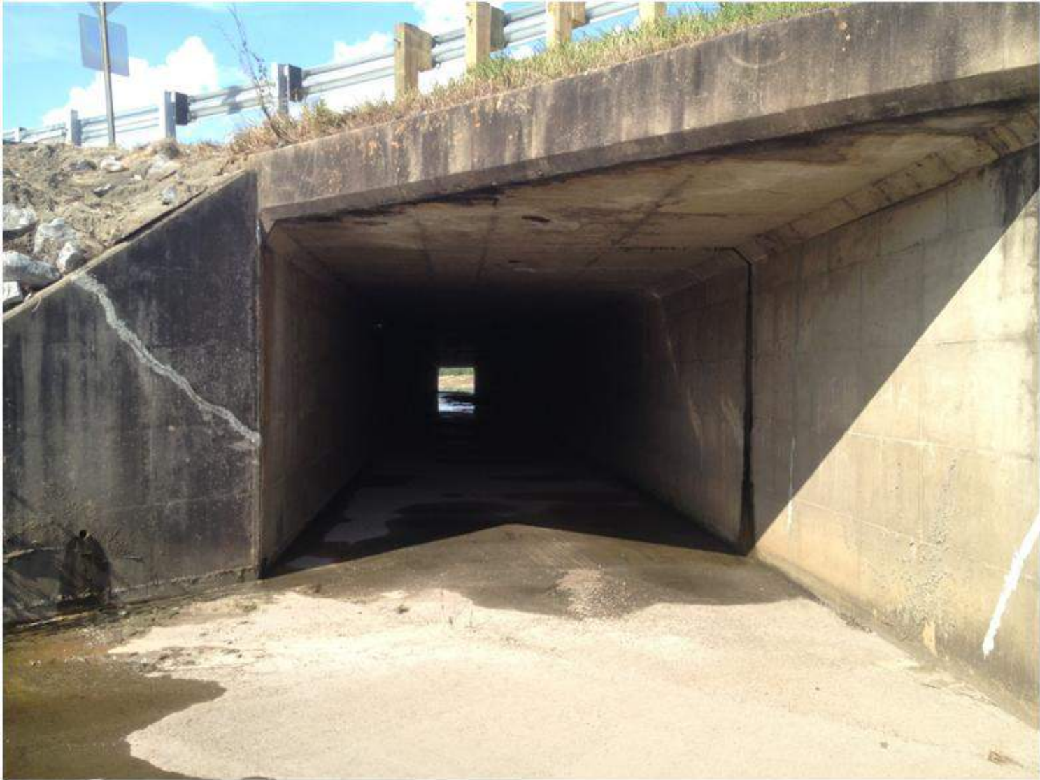
Figure 3-34 Culvert under I-65, a dry cell, may provide an opportunity for pedestrian access in the proposed greenway trail system.
