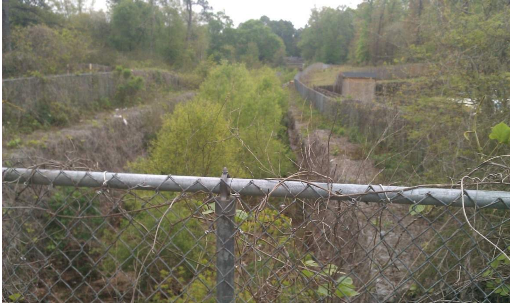
Figure 3-11 Gabion lined channel filled with sediment and vegetation reduces system drainage capacity and can result in localized flooding in the watershed (Location: TWEM downstream of Renn Street)
