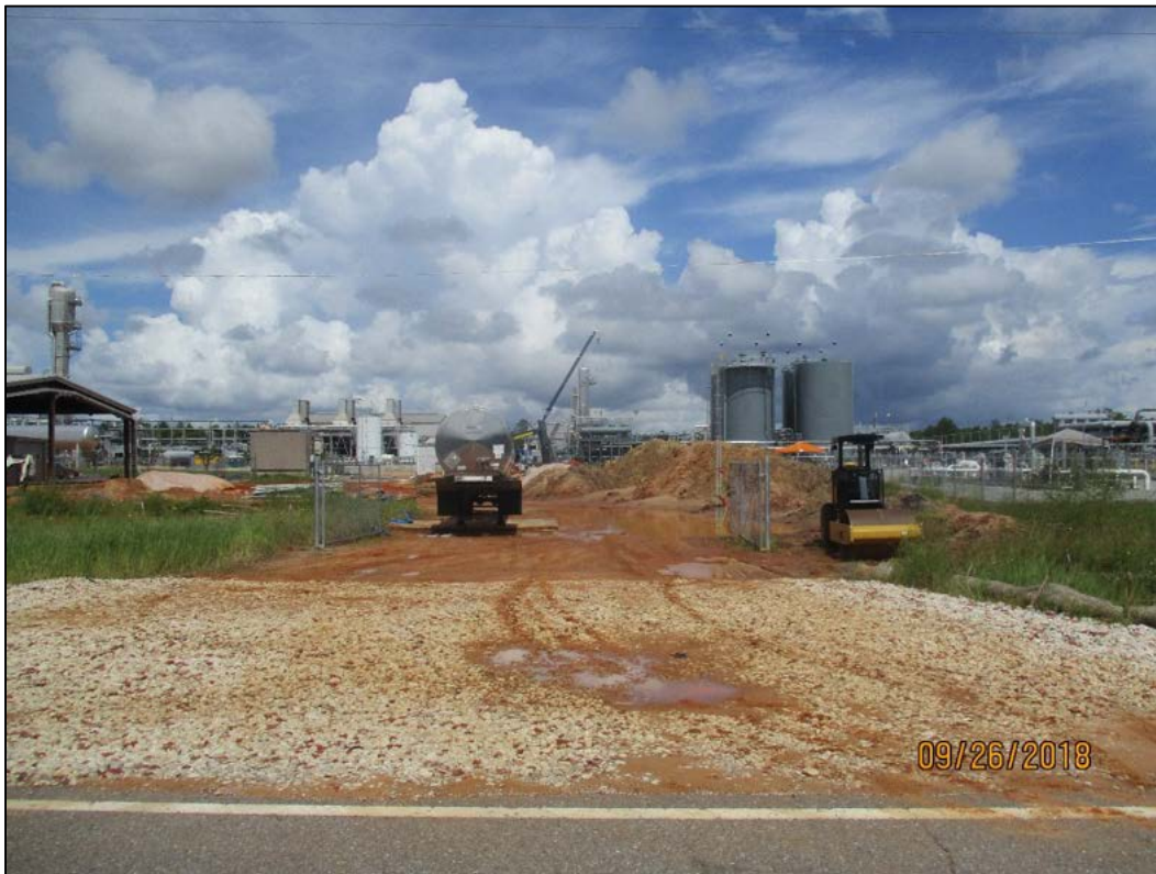
Figure 4.9 Failure to install BMPs in the upper Watershed
