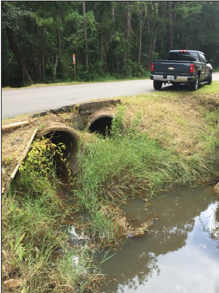
Figure 4.14 Elevated and clogged culvert crossing preventing upstream migration of aquatic organisms
