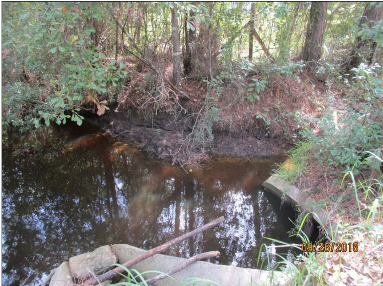
Figure 4.13 Bank scour associated with a road culvert crossing At Saint Michael Road
