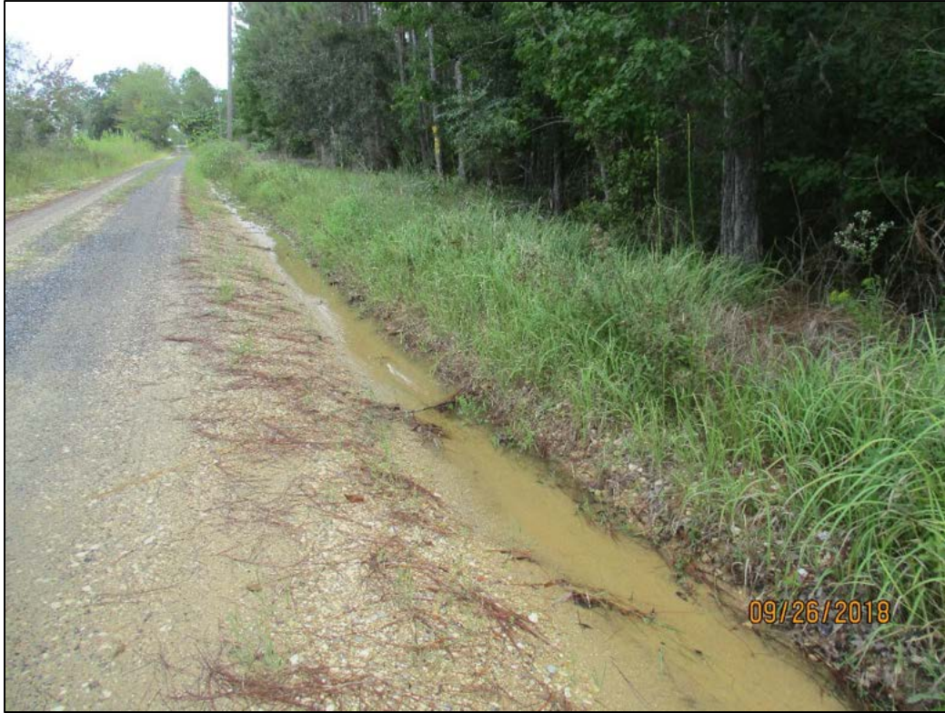
Figure 4.4 Unpaved roads in the lower Watershed
