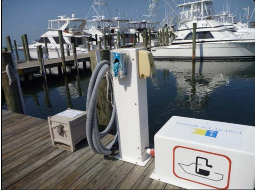
Figure 6.22 Boat pump out station. Source: FDEP Clean Marina Program
